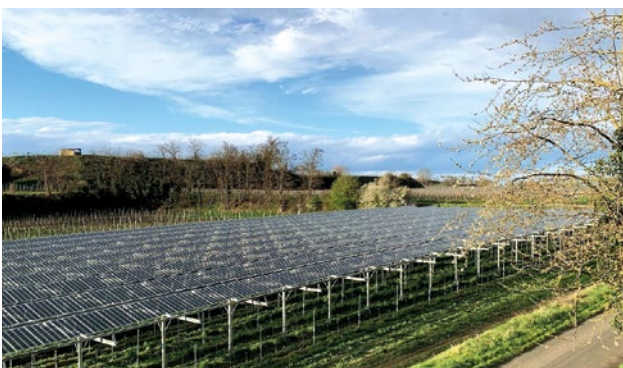
Quelle: Gsun GmbH – Vino Photovoltaik in Freiburg
